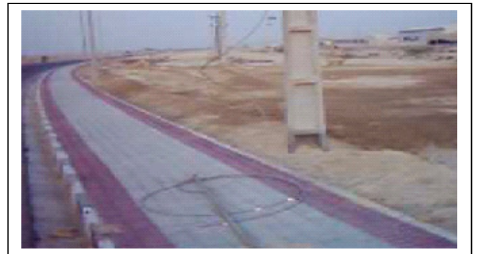
Figure 6. (a) Arcs in HIF test on cement surface
